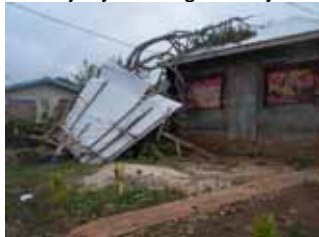
Roofs blown off
